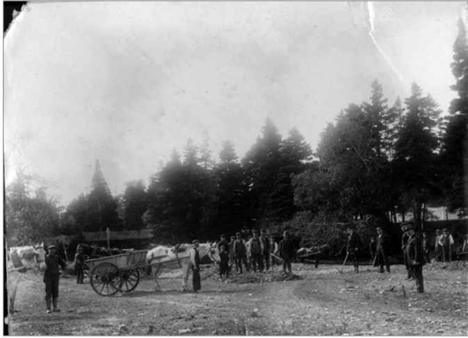
FIG. 11. EXCAVATING THE LAKE AT BOWRING PARK, C. 1913. | ST. JOHN'S, CITY OF ST. JOHN'S ARCHIVES (01-18-018).
