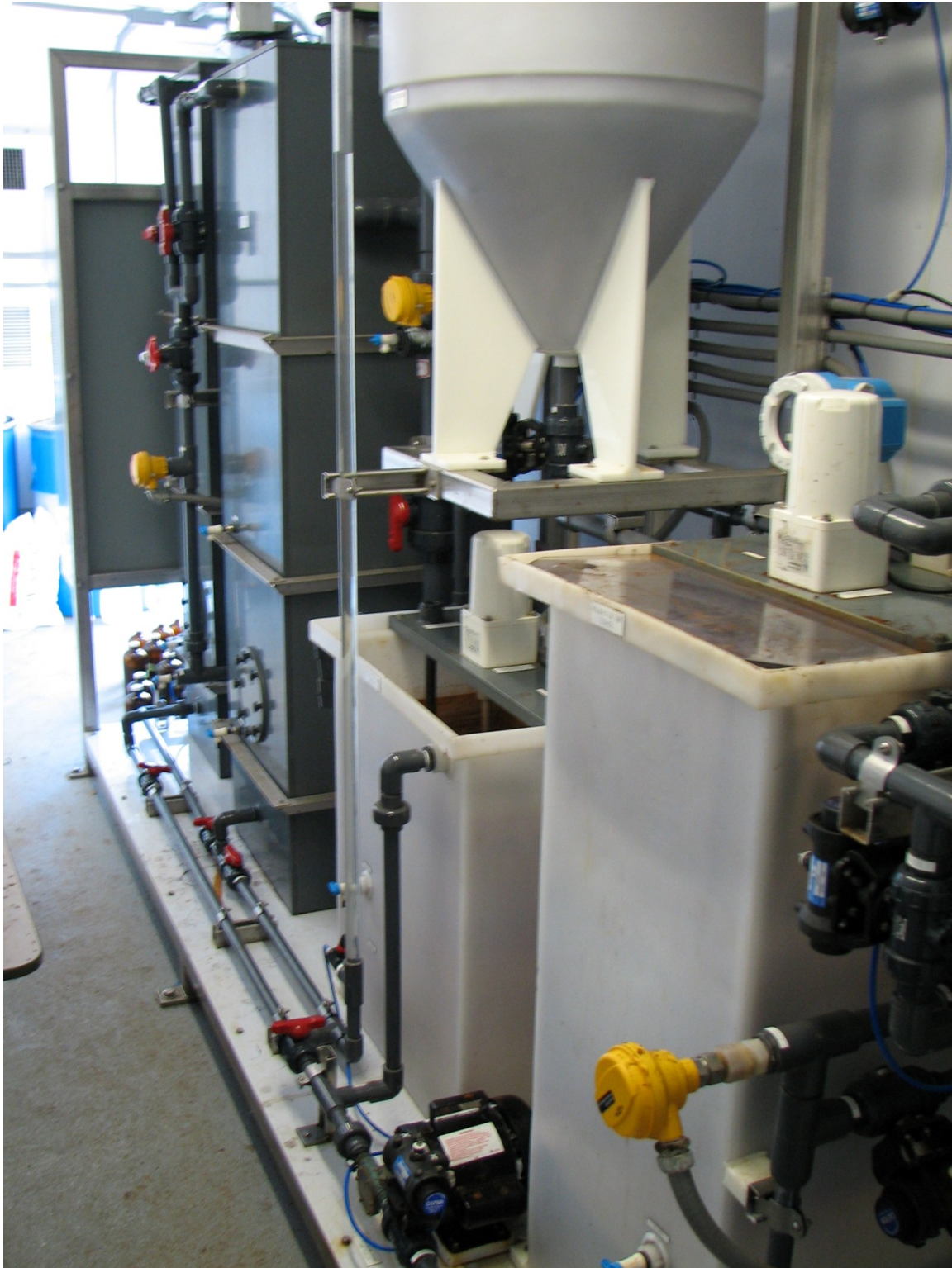
Figure 6.2. On-site photo of 10 USGPM MIEX ® high rate system.
